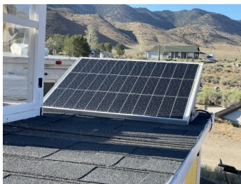
Solar Panel Atop The Post Office
